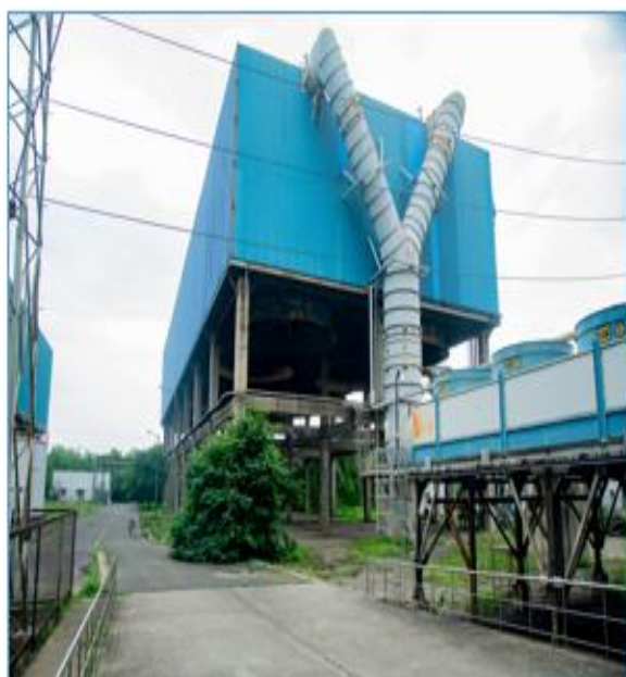
Air Cooled Condenser installed in all the 4 units
